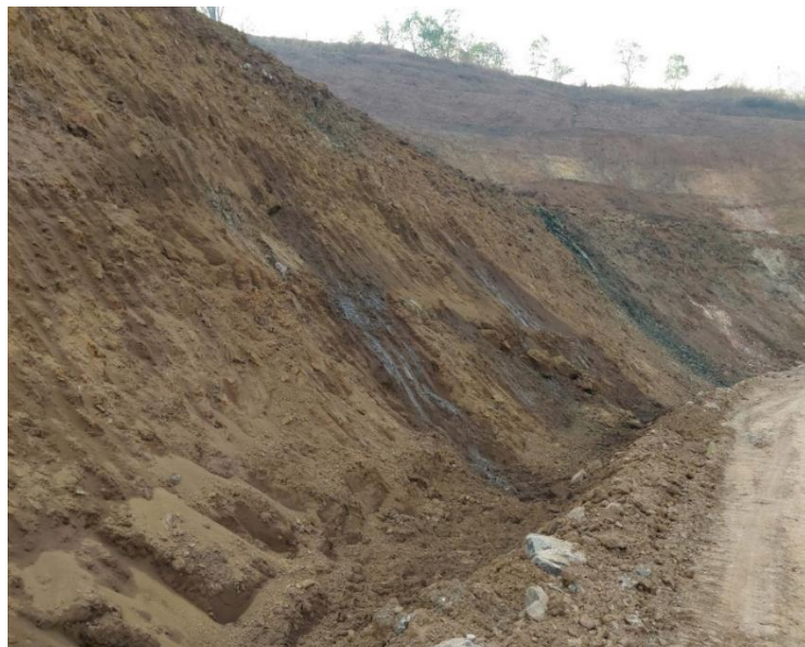
Fig 40: Water seepage from several places of slope wall
