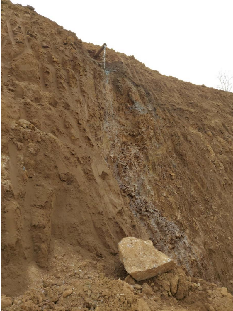
Fig. 39: Water seepage from slope wall
