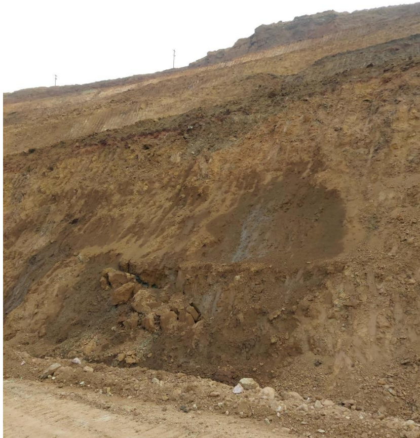
Fig 41: Moist slope wall due to presence of water in slope.
