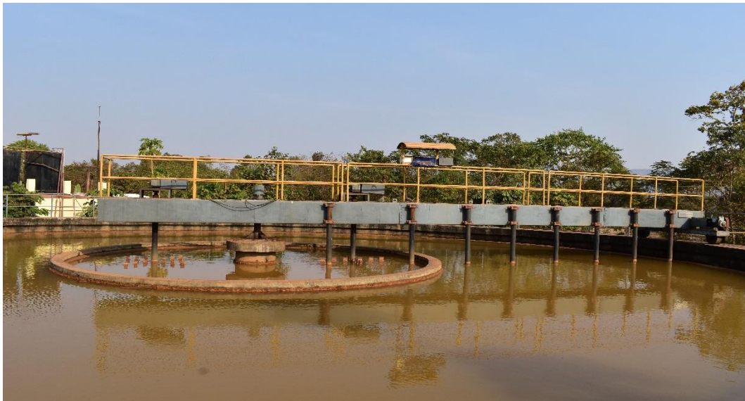
Effluent Treatment Plant for treatment of Mines Seepage Water
