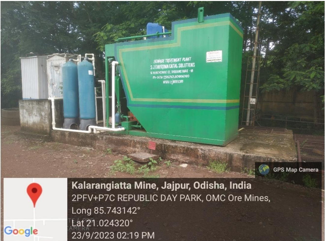
Sewage Treatment Plant for treatment of Domestic Waste Water
